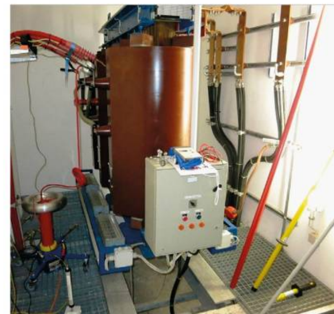
Figure 9. PD measurement setup on a 20 kV / 2 MVA cast-resin transformer
