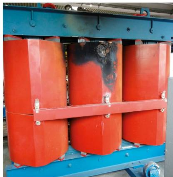
Figure 7. Breakdown fault on cast-resin transformer
