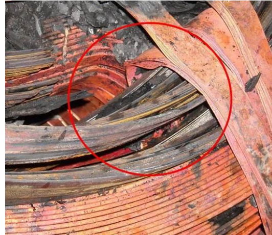
Figure 9 Damaged LV winding
