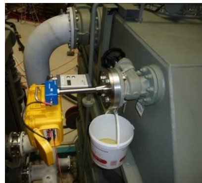
Figure25 UHF sensor mounted on the main drain valve
